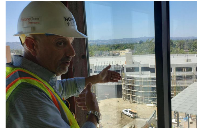
Bisnow/Joseph Pimentel JLL's Patrick Church gives a Bisnow reporter a tour of the construction of Merlone Geier's NoHo West project in North Hollywood.
